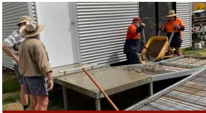
Job seekers build a wheelchair-accessible ramp for the new toilet and shower block behind Blackall’s Lost Art Centre.
